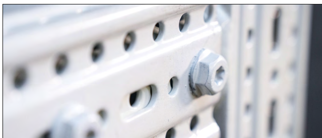
FLS acoperit corect
